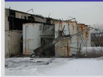
Figure 1. North side of ASCO facility. Damage to building 46 and debris around the decant water tanks.
