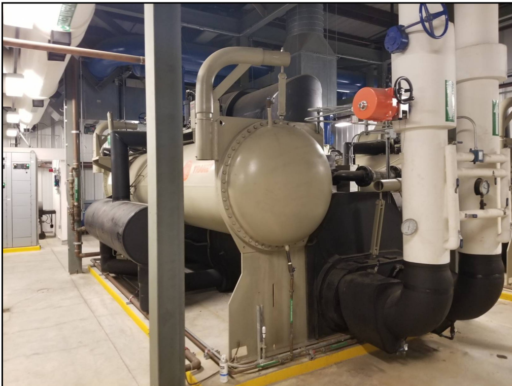
54 : View of a typical chiller.
