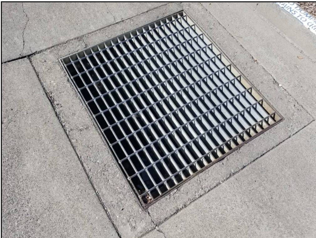
68 : View of a typical storm drain inlet in the site parking lots.
