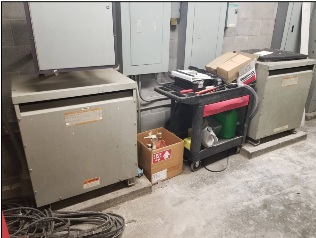
62 : View of two typical interior transformers. No signs of leaks or spills were observed.
