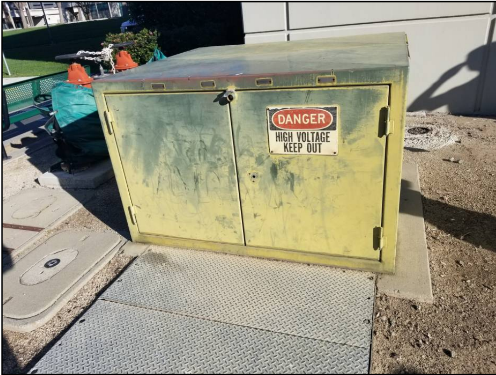
69 : View of a typical pad-mounted transformer on the site. No signs of leaks or spills were observed.
