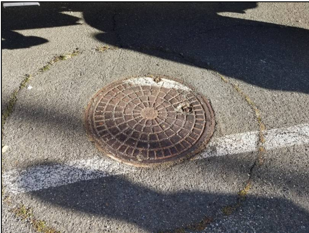
66 : View of one of the grease interceptors on the site.
