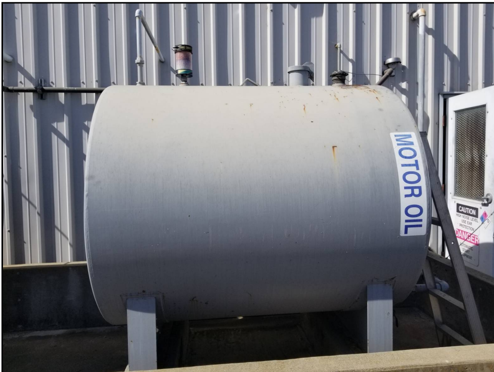
58 : View of the 1,000-gallon oil AST. No signs of leaks or spills were observed.
