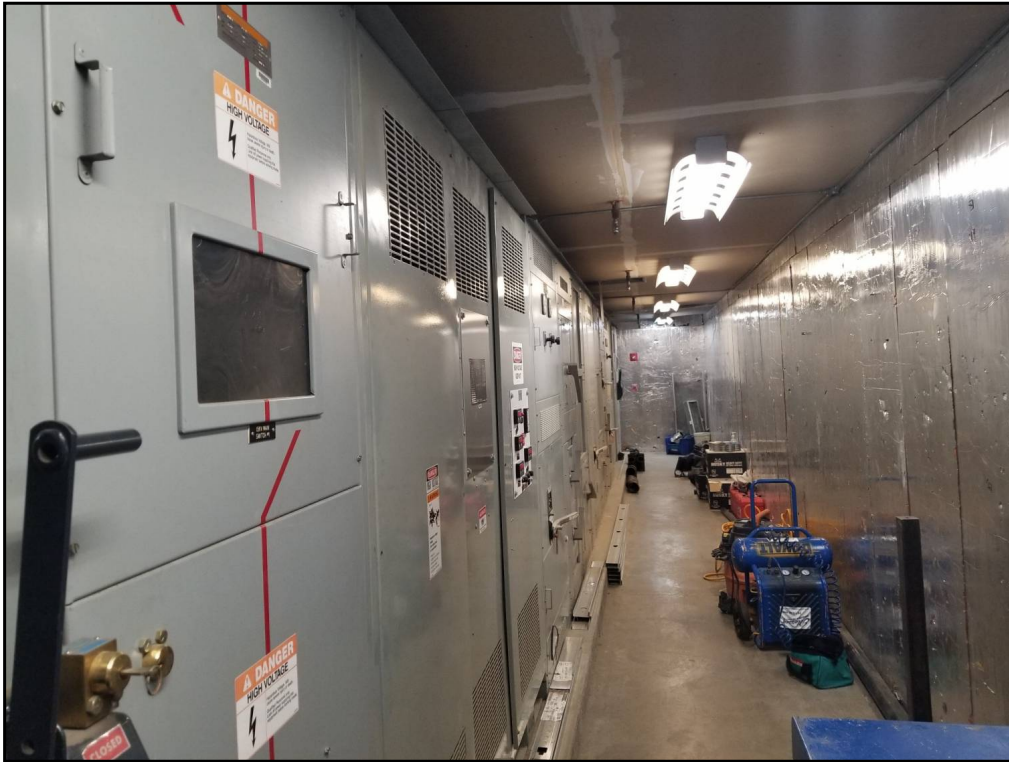
61 : View of a typical building electrical room.
