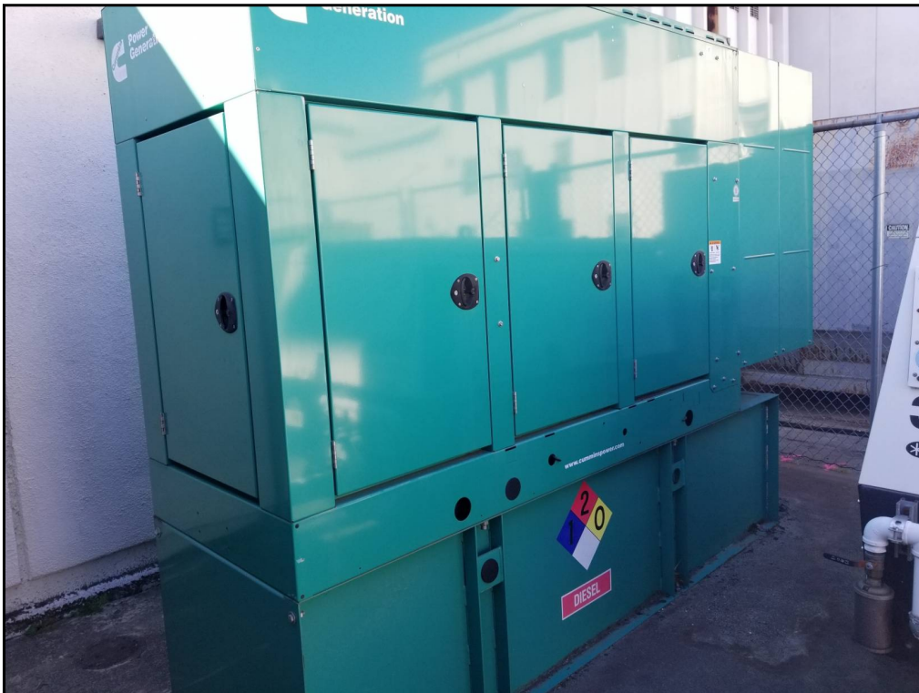
64 : View of one of the generators with a 350-gallon diesel belly tank. No signs of leaks or spills were observed.
