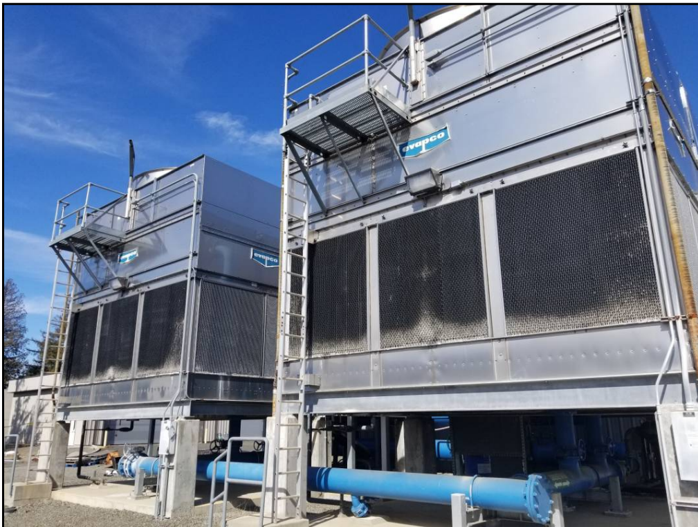
56 : View of a typical cooling tower.
