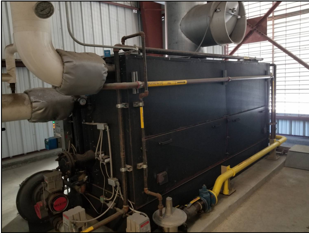
55 : View of a typical boiler.
