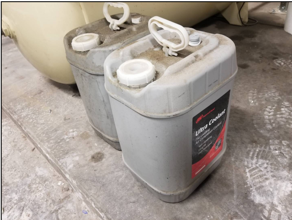
72 : View of two containers of air compressor coolant.
