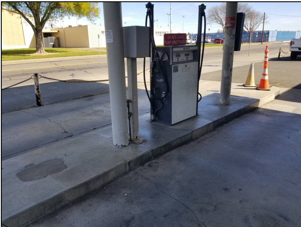
36 : View of the pump island.
