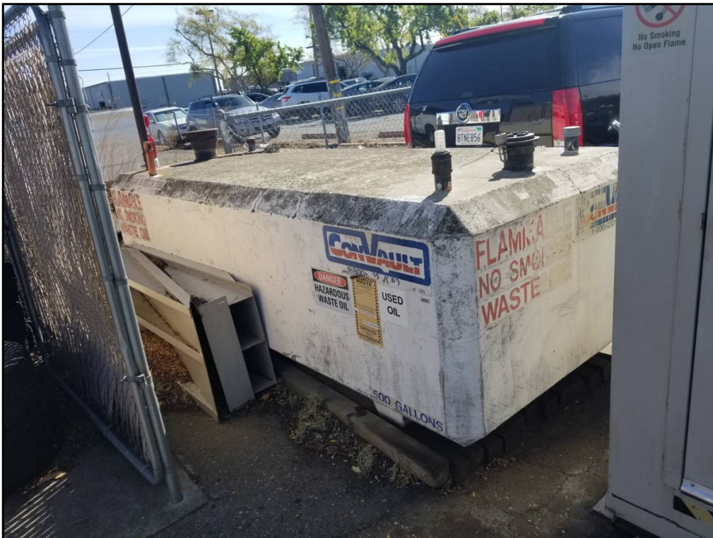
38 : View of the 500-gallon waste oil AST.
