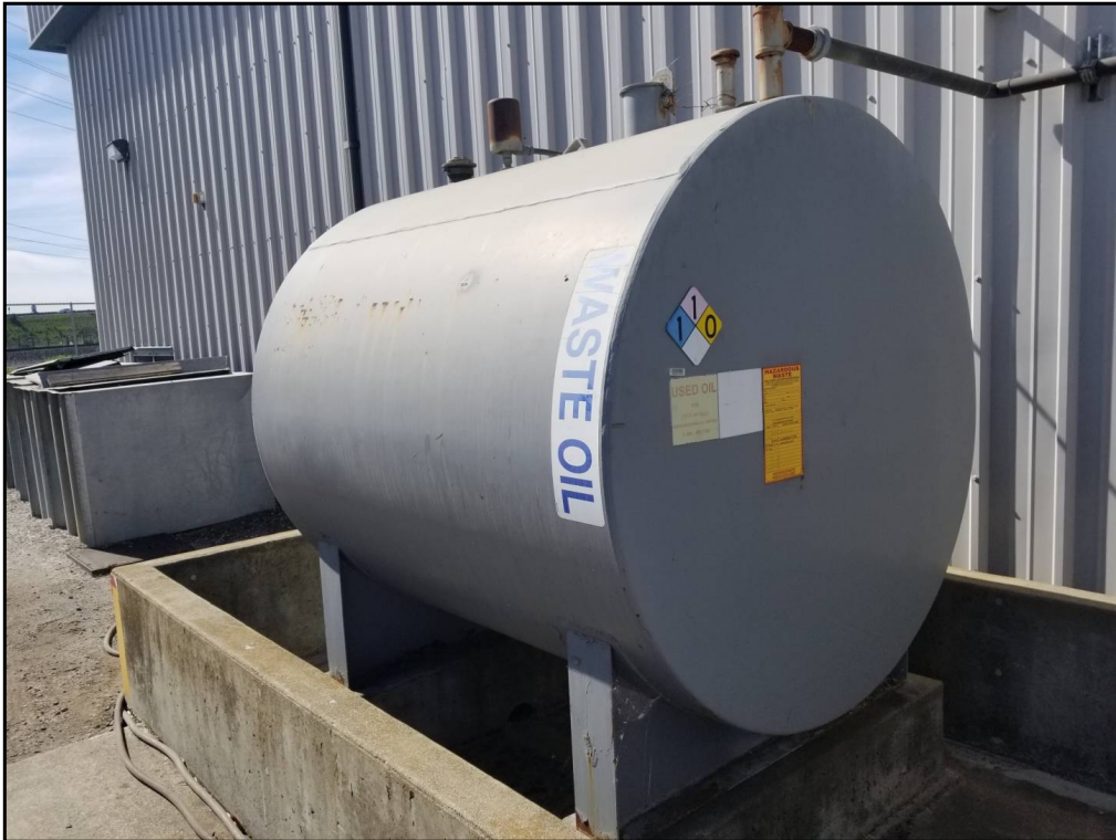
59 : View of the 1,000-gallon waste oil AST. No signs of leaks or spills were observed.
