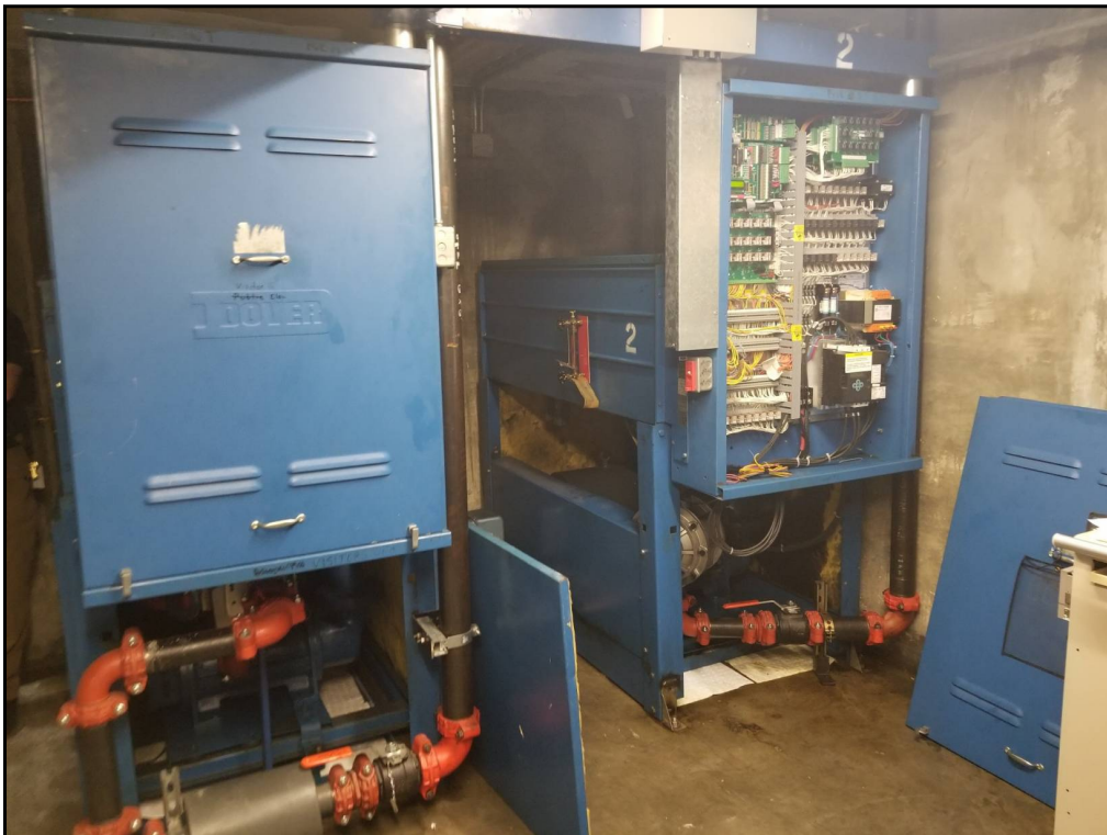
18 : View of a typical elevator mechanical room. No signs of leaks or spills were observed.
