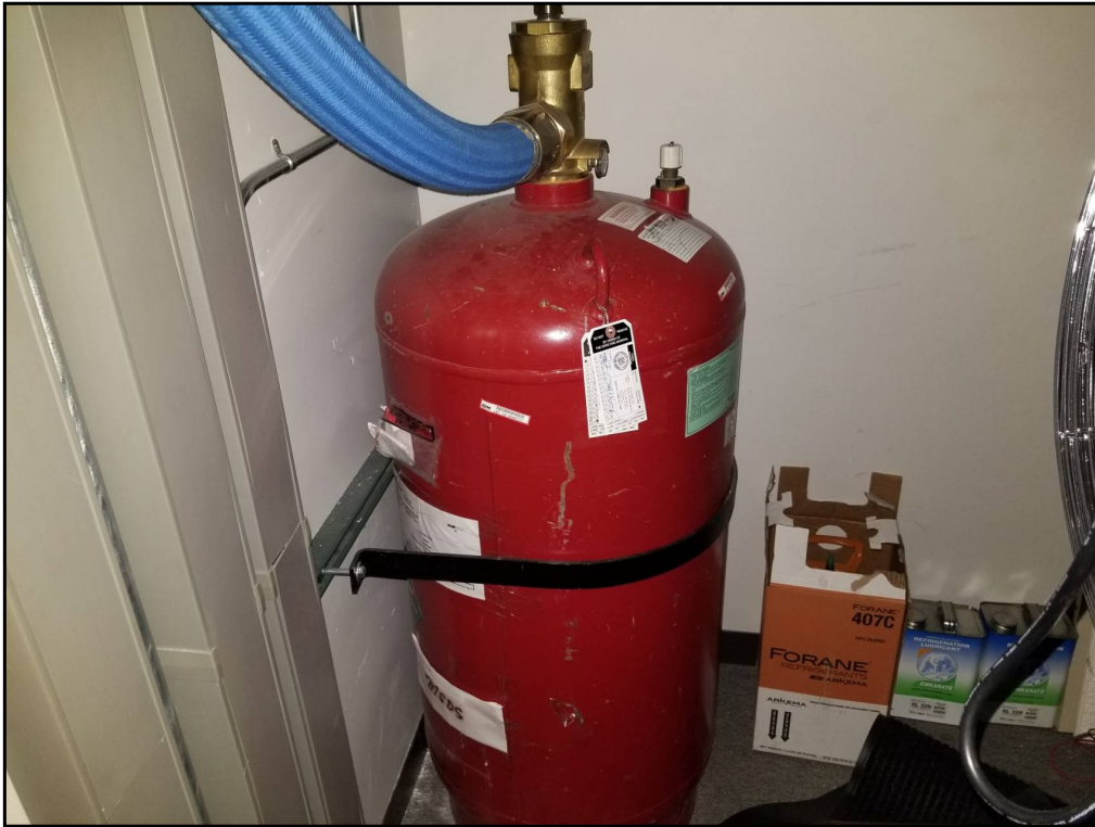
73 : View of a typical fire suppressant tank. No signs of leaks or spills were observed.
