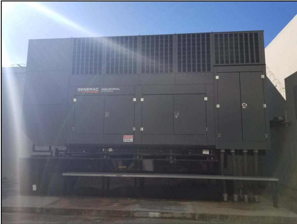
65 : View of the generator with a 2,310-gallon diesel belly tank. No signs of leaks or spills were observed.
