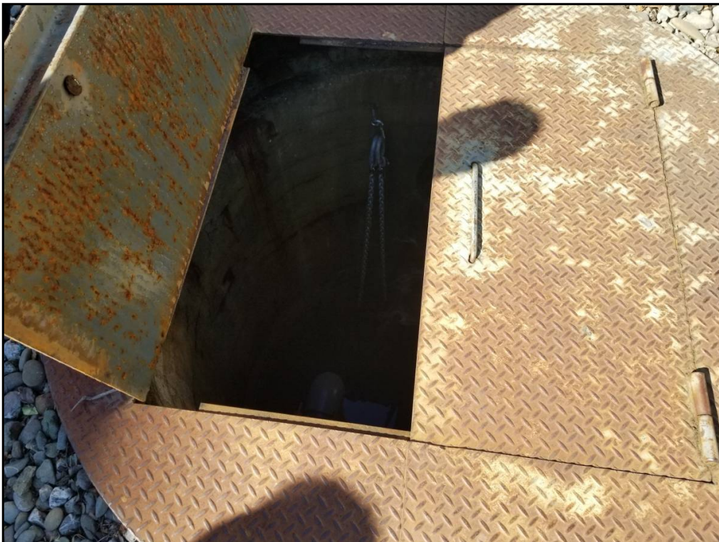
70 : View of a typical sump.
