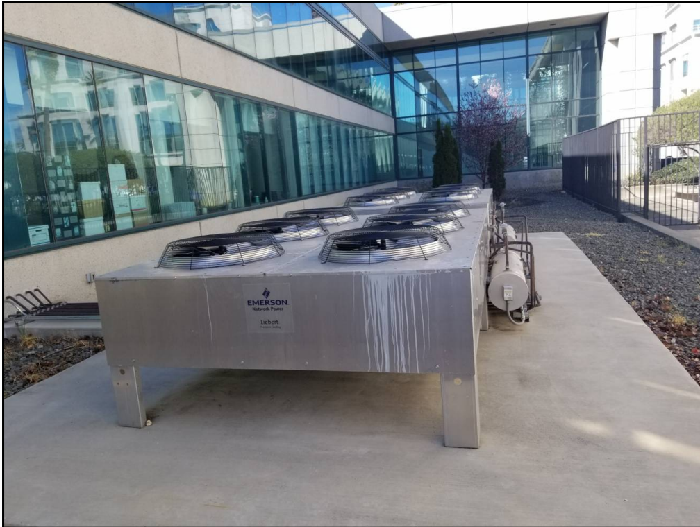
71 : View of typical HVAC units.
