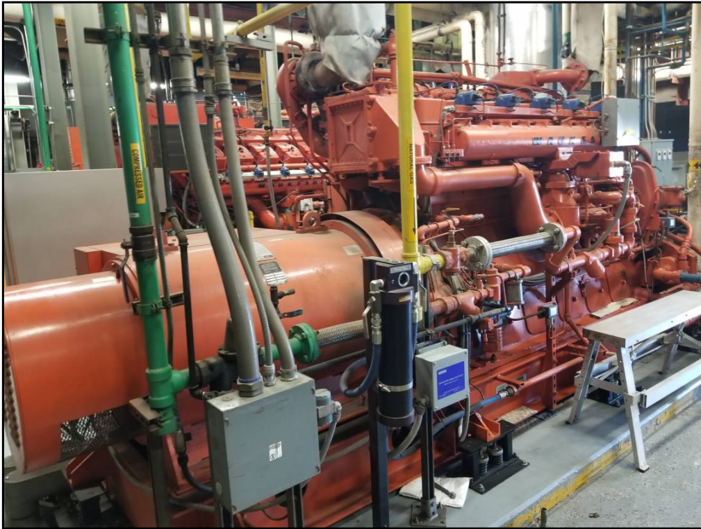
57 : View of a typical natural gas generator.
