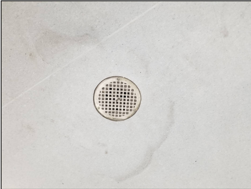
67 : View of typical floor drain.
