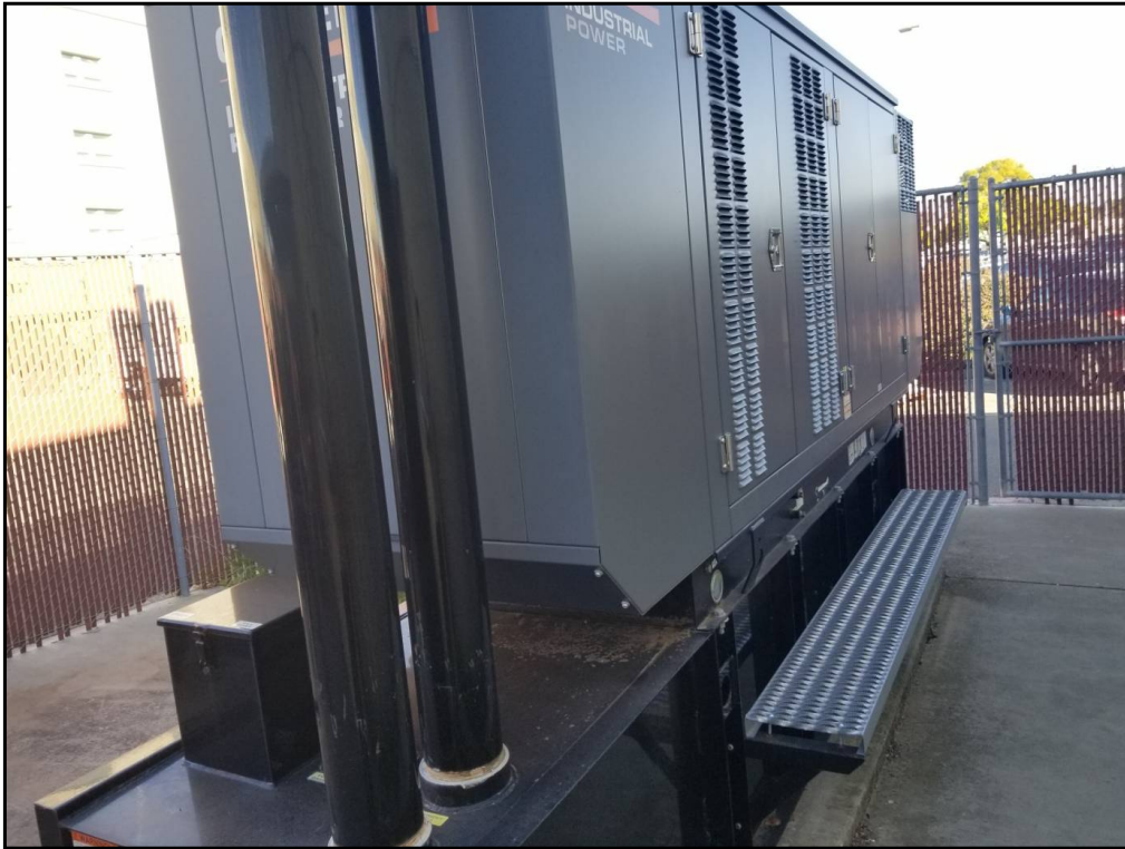
63 : View of one of the generators with a 350-gallon diesel belly tank. No signs of leaks or spills were observed.
