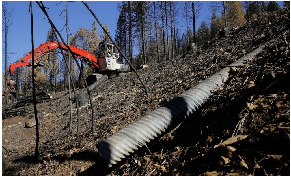
Figure 4-62: Landslide Prevention Post-Wildfire Source: The San Francisco Gate
