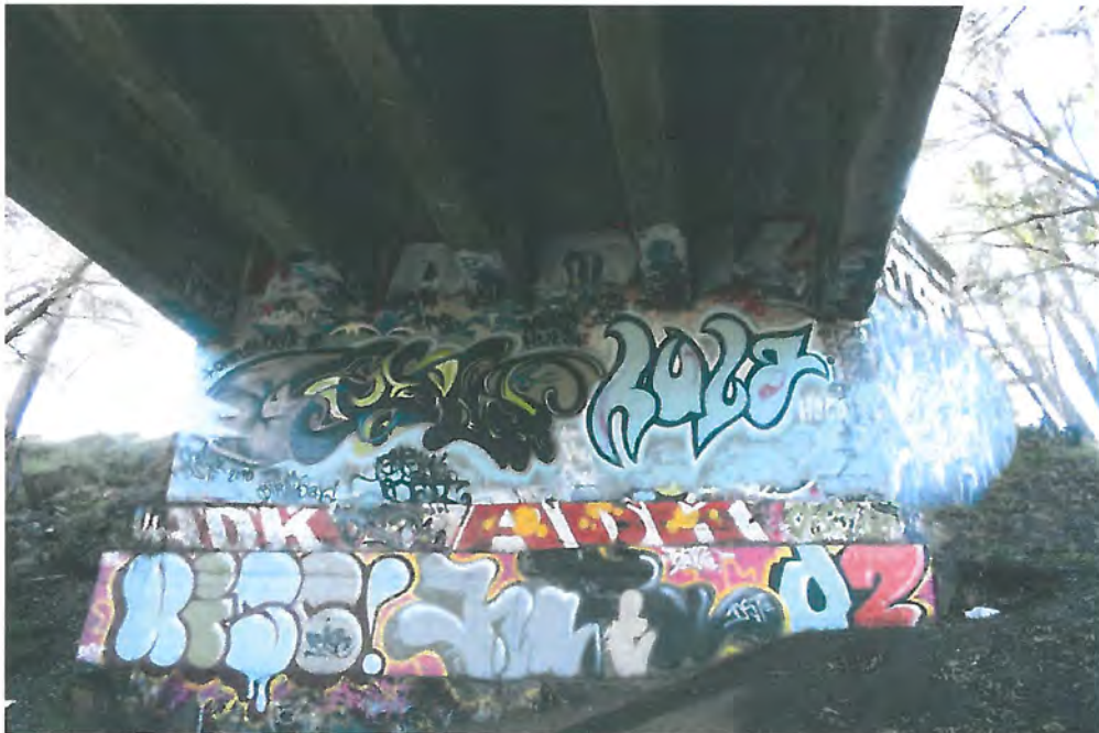
Image 5. South abutment, U-shaped abutment with graffiti, view facing south.
