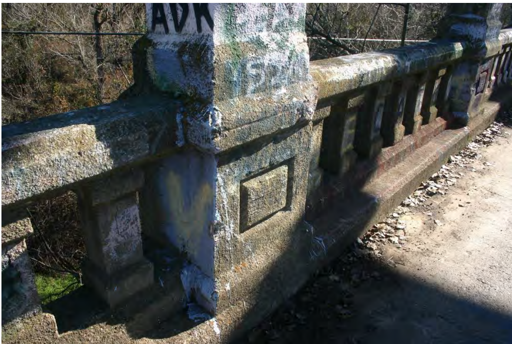
Photograph 4. Character-defining aesthetic features include an open reinforced concrete railing, integrated between the vertical hangar columns that connect the arches and longitudinal girders. Detail view.
