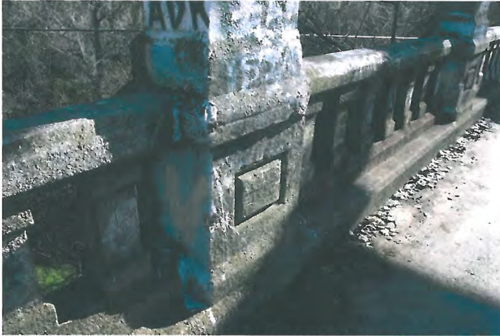
Image 4. Reinforced concrete railing with rectangular window rail design and smooth concrete finish, view facing southeast.
