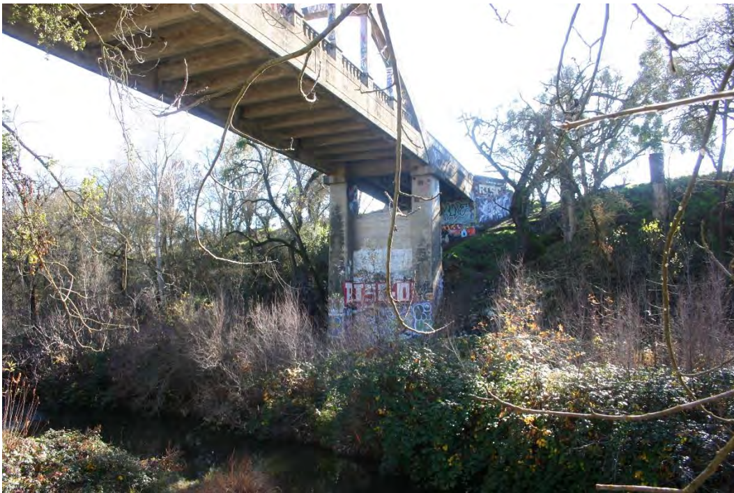
Photograph 6. Exterior girders may be strengthened by adding interior girders. These changes will not be visible to pedestrian or motorists that use the bridge. View facing southeast.
