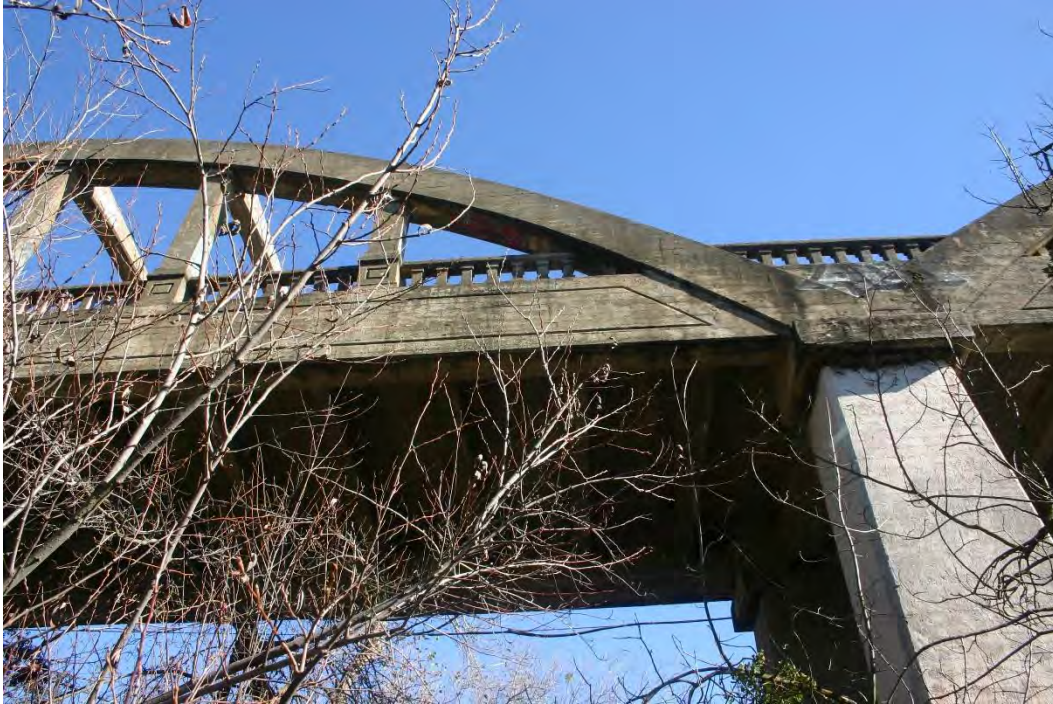
Photograph 3. Character-defining structural features include reinforced concrete arches tied to reinforced exterior longitudinal girders; reinforced concrete overhead braces that connect the arches; and vertical hangar columns that connect the arches to the longitudinal girders. Detail view.
