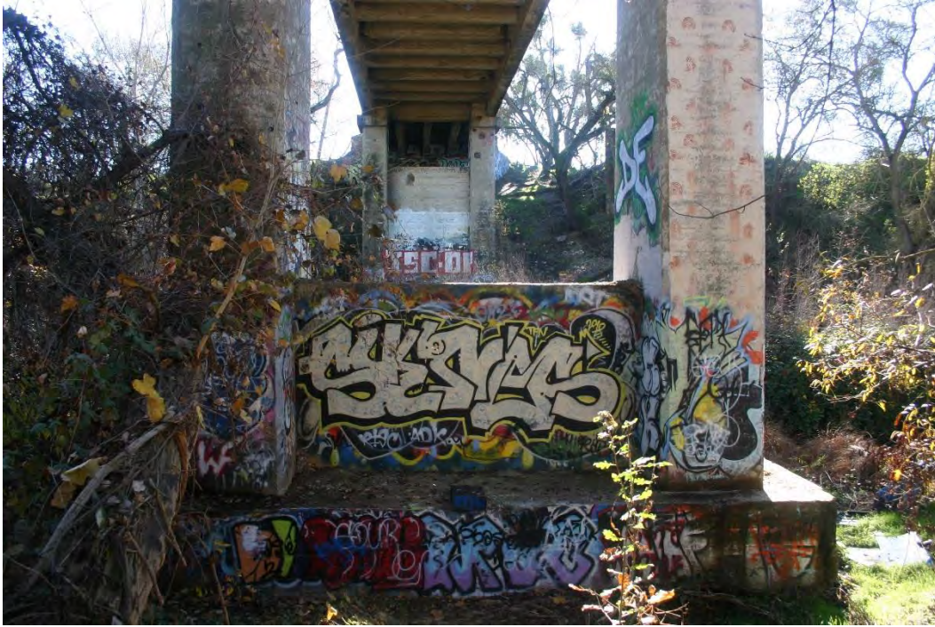
Photograph 7. Pier columns will be fiber wrapped and filled in with reinforced concrete shear walls. The piers are already partially filled in and adding a shear wall in between the pier columns would not detract from the character-defining structural and aesthetic features on the superstructure. View facing south.
