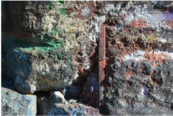
Figure 9 - Exposed rebar at east Abutment 1 railing
