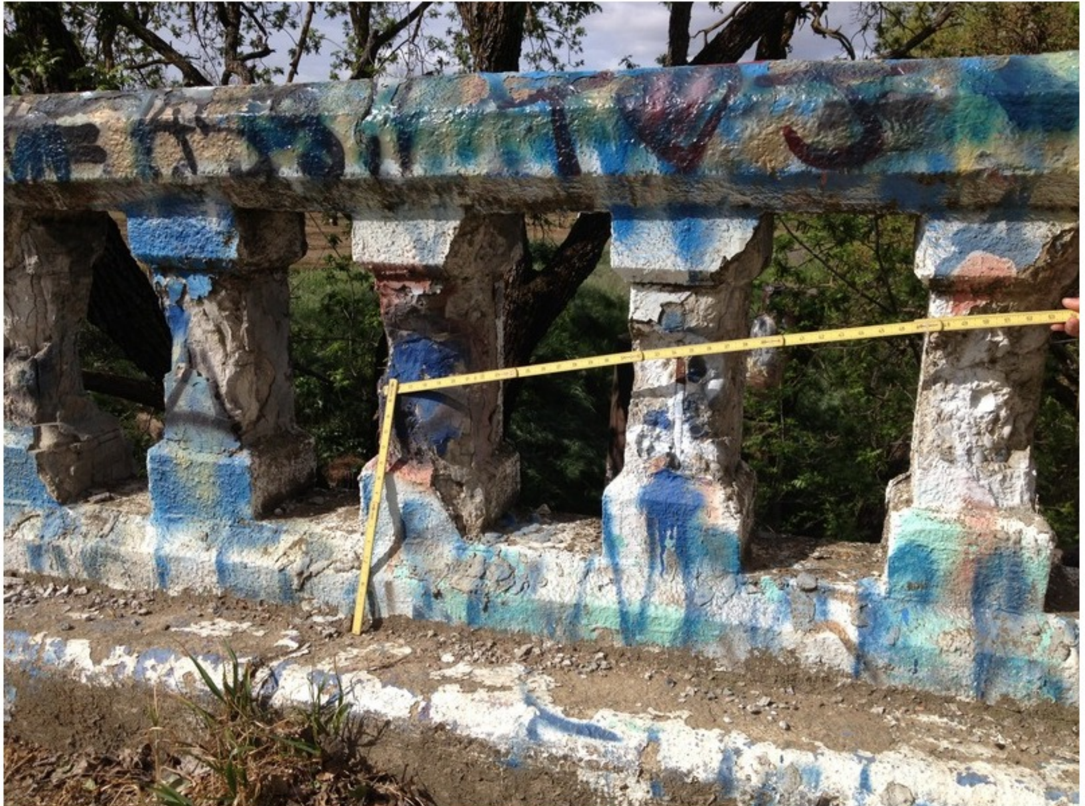
Photo No. 1 Damage to the left rail in Span 1
