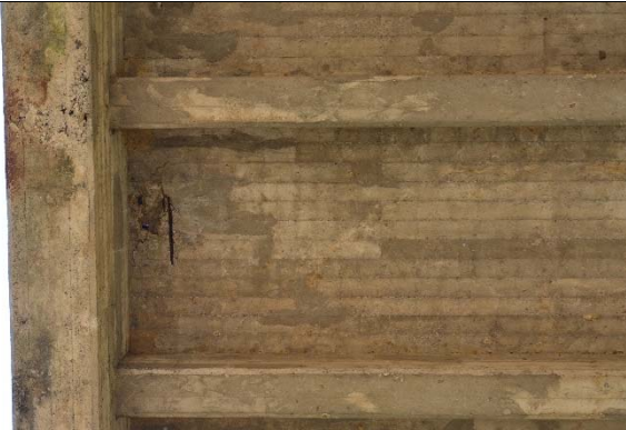
Figure 19 - Unnumbered Defect (DSC_428) Bay 6
