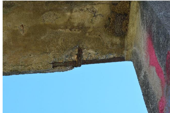
Figure 10 - Spalled overhead section of arch
