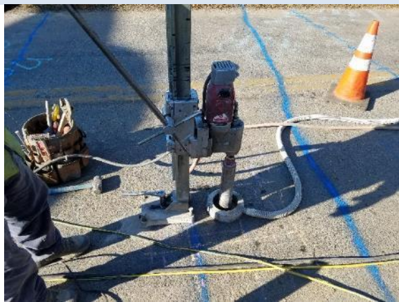
Figure 37 - Bridge Deck at Pier 4/Abut 5 (Core 3)
