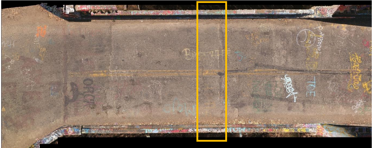
Figure 7 - Location of crack between Abutment 1 and Pier 2 as shown through UAS image
