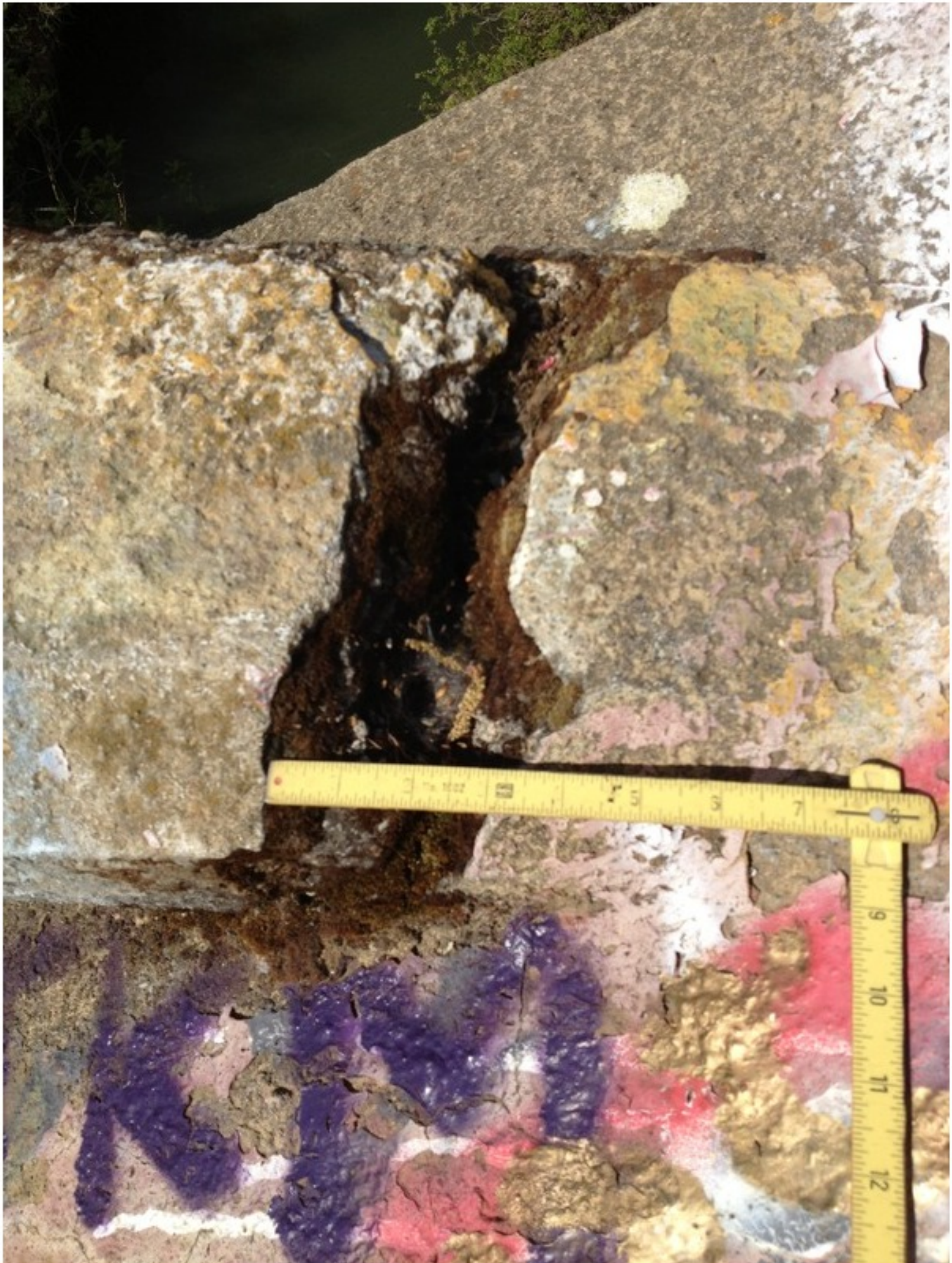
Photo No. 2 Crack on the left rail at the connection with the northern arch over Bent 3
