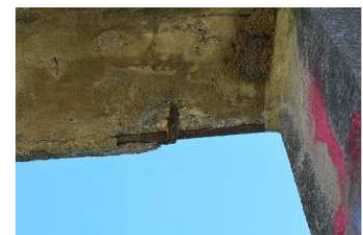
Figure 10 - Spalled overhead section of arch
