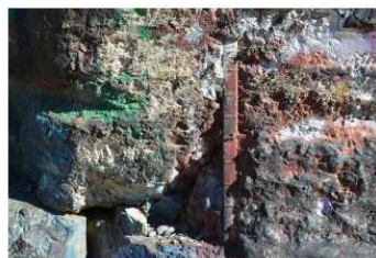
Figure 9 - Exposed rebar at east Abutment 1 railing
